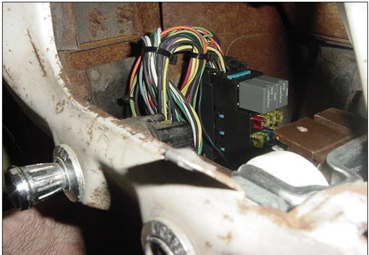
Figure 3 Fuse Block Position
